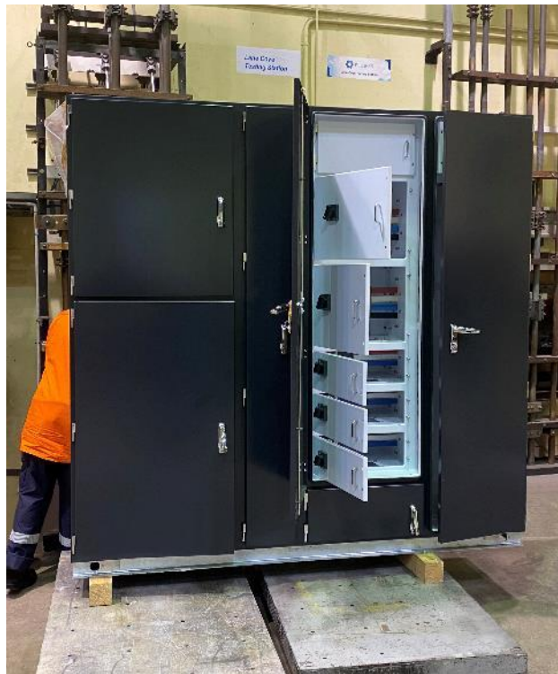
Fuji SMBE Macquarie's tough new outdoor switchboard at the testing facility in NSW
